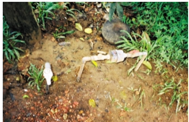
A water meter set in each household
